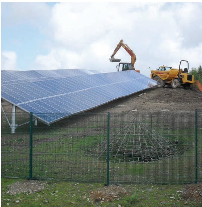
Figure 5 Construction of a 1.4MW solar farm at the former tin mine site at Wheal Jane, Cornwall. Such sites should generally be considered for such development in preference to agricultural land.
