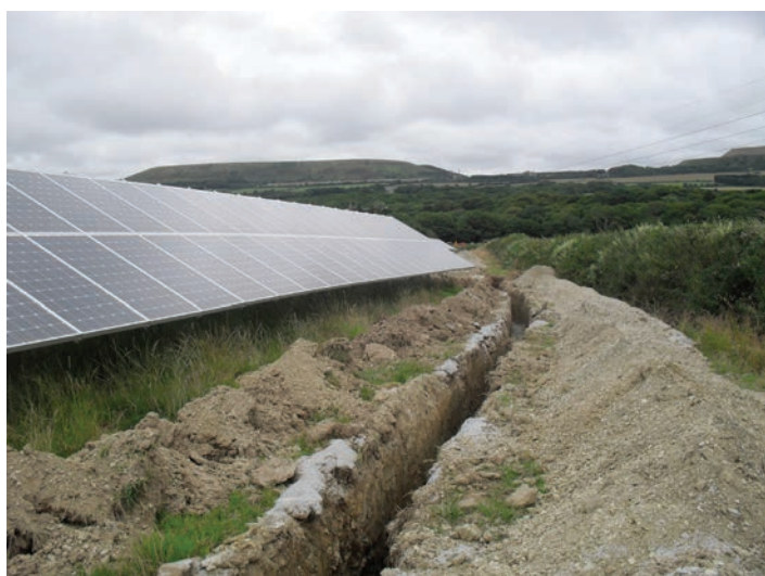
Figure 9 Soil excavation during cable trenching at the 5MW Trefullock solar farm in Cornwall. Note how topsoil and subsoil are stored on opposite sides of the cable trench in order to avoid the mixing of soil types and facilitate subsequent soil replacement and site restoration.
