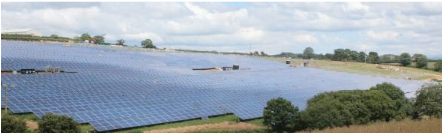
Figure 26 Howton 5MW solar farm, Cornwall. Image courtesy of Low Carbon Solar Partners.
