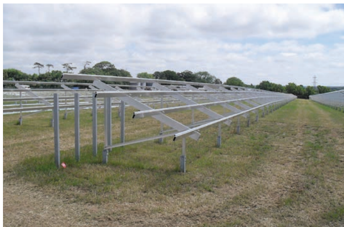
Figure 14 The ground anchors and framework associated with the development of the 1.4MW Benbole solar farm in Cornwall.
