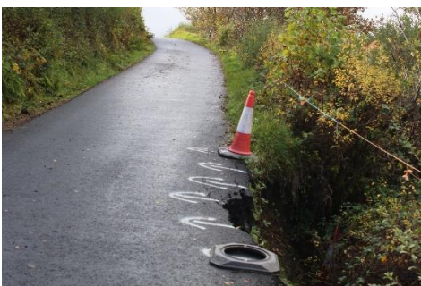
Flood Damage – Liggins Road [Coneyglen] This year 2018
