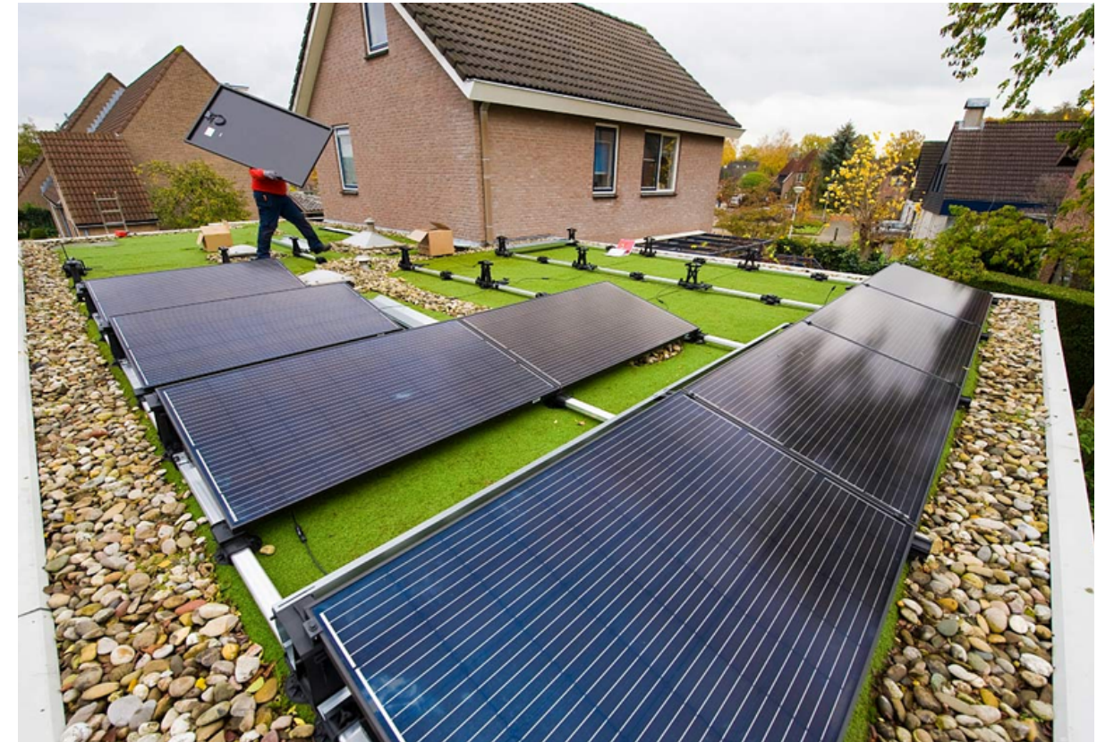
Roof mounted solar panels on a flat roof
