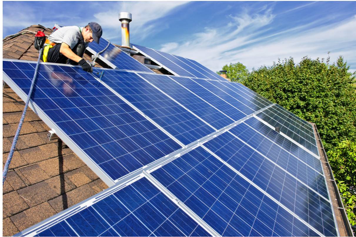
Roof mounted solar panels on a pitched roof
